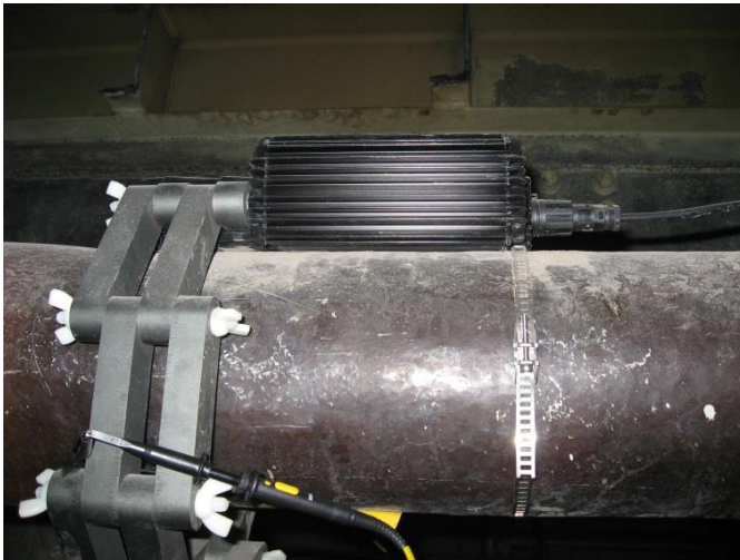
30' before the E1 shower nozzles
