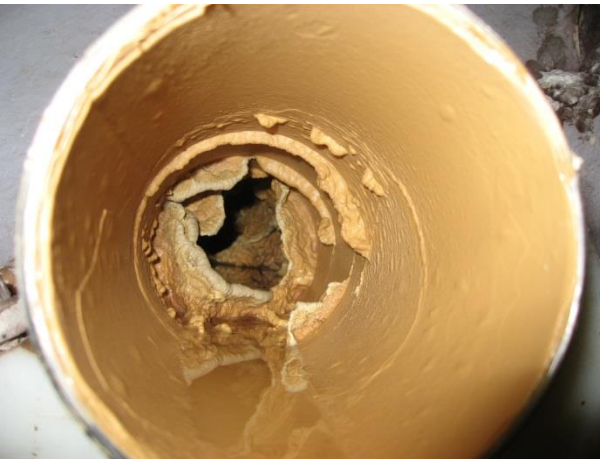
Untreated D1 nozzle – close up
