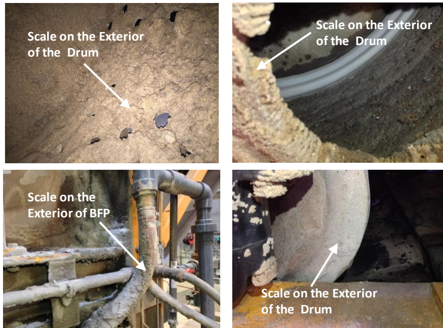
Figure 4: Baseline Condition Before Energizing HydroFLOW
