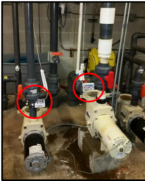
Two HS48 units on Hot Tub and Wader Pools
